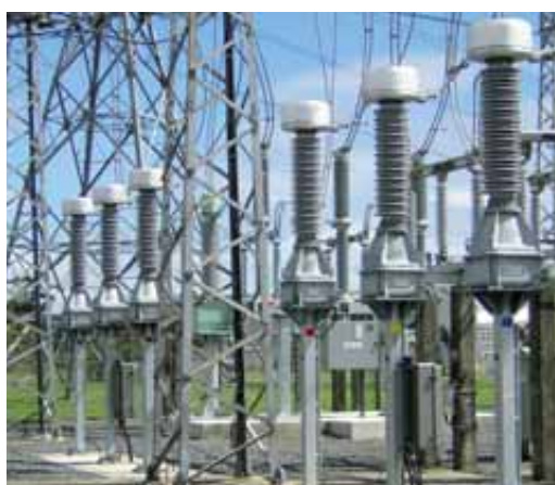
2. 123 kV Inductive voltage transformers. Transpower (New Zealand).
