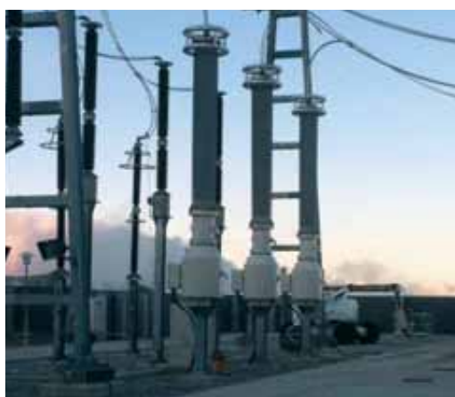
4. 420 kV Inductive voltage transformer. R.E.E. (Spain).
