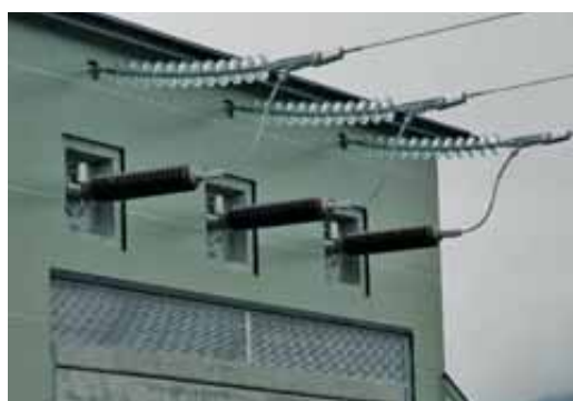
> Indoor/outdoor wall-bushing in a distribution substation.
