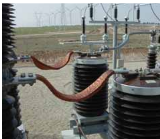
> 72.5 kV Current transformer (CX) used for wind farm substation protection. Iberdrola (Spain).
