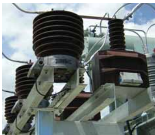
> 36 kV Current transformers (CR) and voltage transformers (UR). Revenue metering. Electronet Services (New Zealand).
