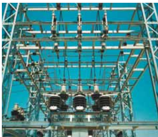
> 24 kV Current transformers (CX), protection for substation. Iberdrola (Spain).
