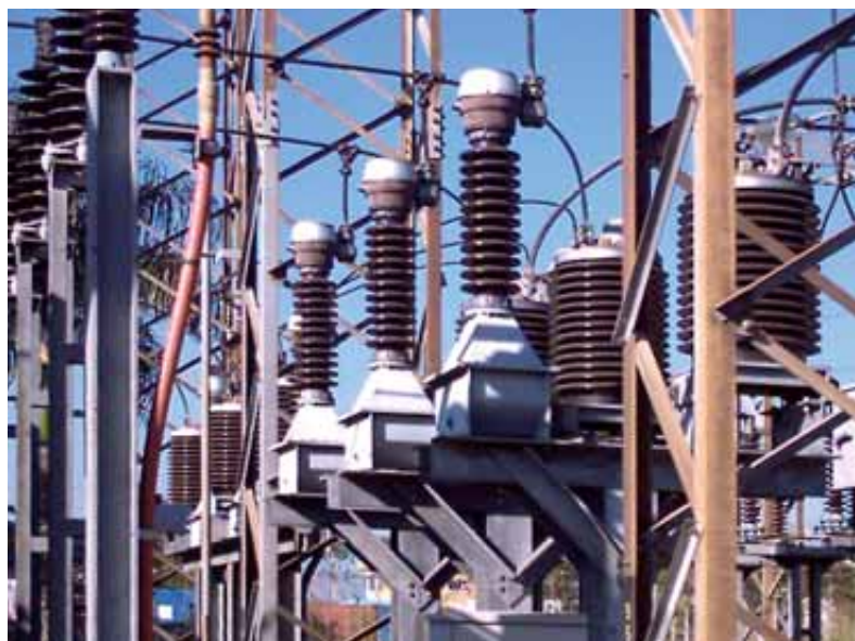
> 36 kV UZK Transformers. Transpower (New Zealand).
